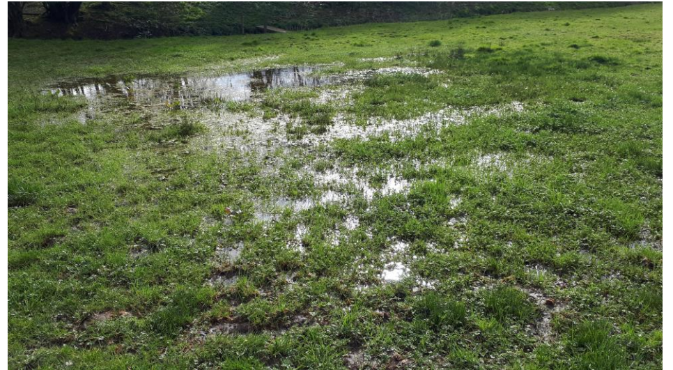
G201 _ seepage on northern banks of churn tributary looking S
