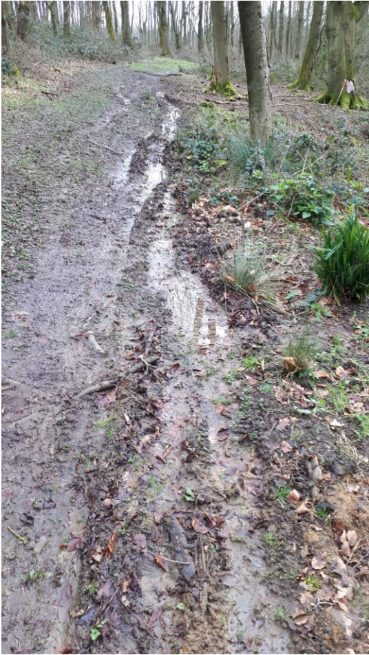
G180a _ seepage at Rushwood Kennels looking N
