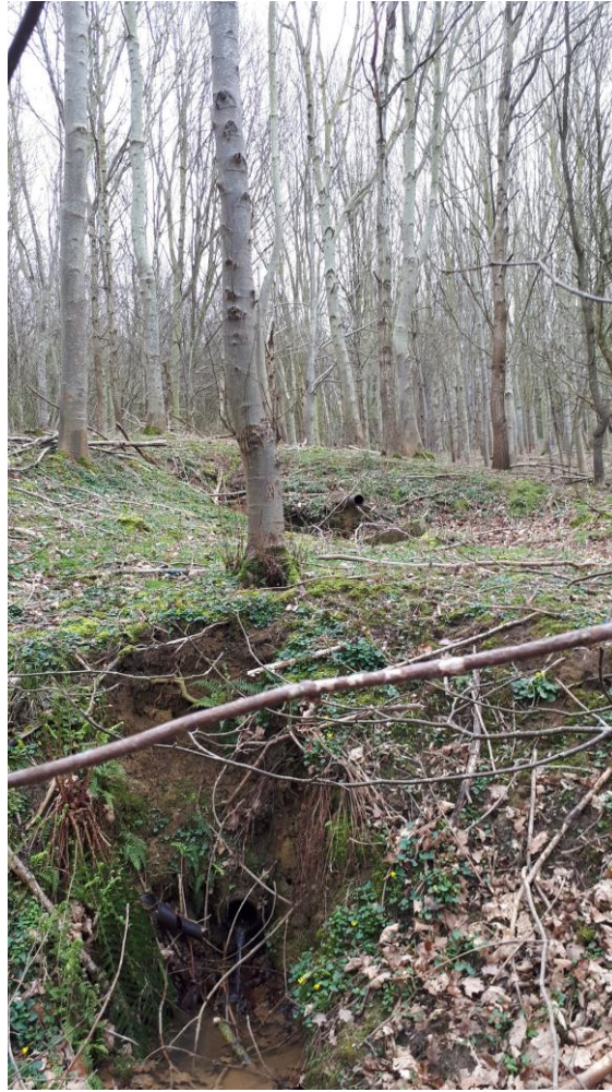
G192 _ exposed pipes used for managing spring flows upper pipe is dry looking N
