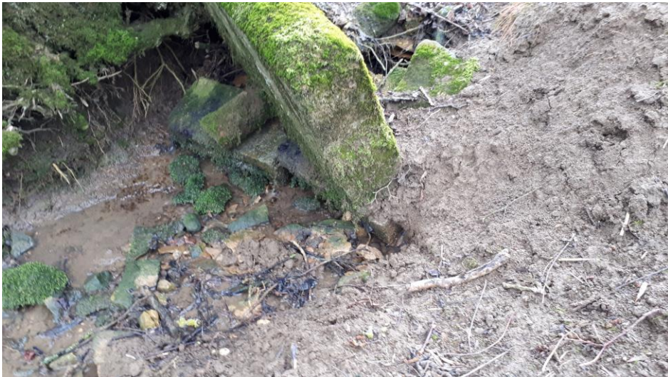
G177 _ broken piped spring, possible overflow or land drainage from field
