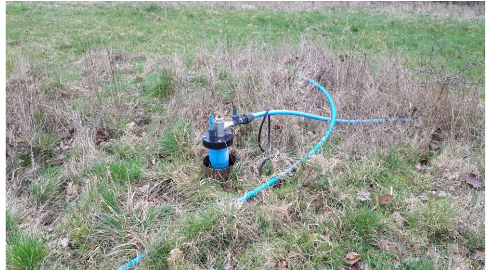
G205 _ abstraction borehole on golf course grounds not used, but intended for top up
