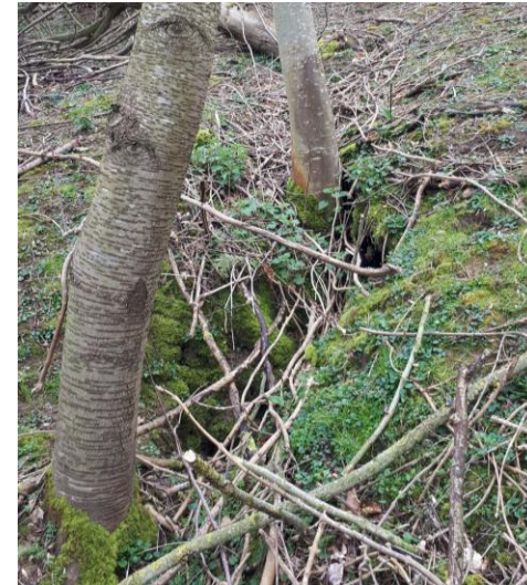
G190 _ staggered re-emerging spring flows exposed by collapse of ground by trees looking N
