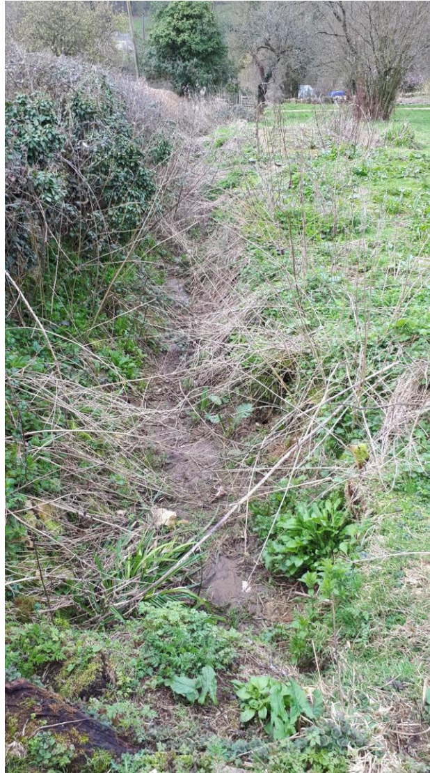
G223 _ land drainage flowing to road drains farm area and some seepage, damp with no flow looking SW DS
